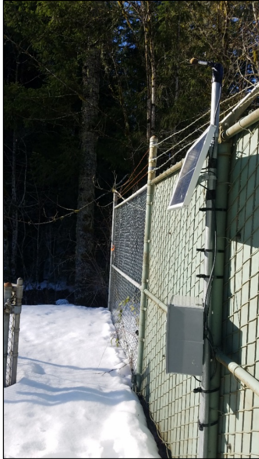
A solar powered acoustic bat call recording unit
