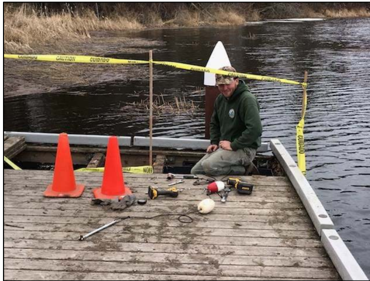
Natural Resource Technician Deyo repairing ice damage to the Lake Terrell boat launch dock
