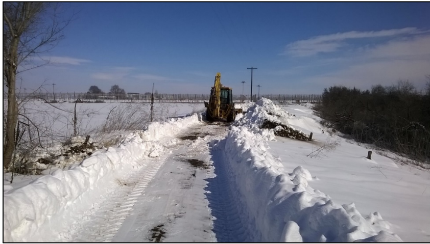
Using the backhoe to clear snow from the Giffen Lake access road
