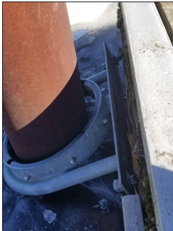
Ice damage to Lake Terrell boat launch dock
