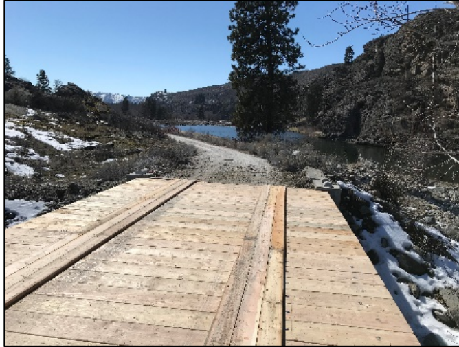
Bridge Deck Replacement leading into the McLoughlin Falls Unit – Photo by Wehmeyer
