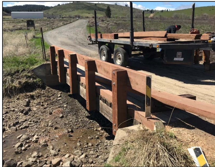
New rails on bridge across Kittitas Reclamation District canal in Joe Watt Canyon
