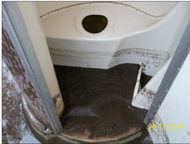
High water mark inside fiberglass restroom along Joseph Creek
