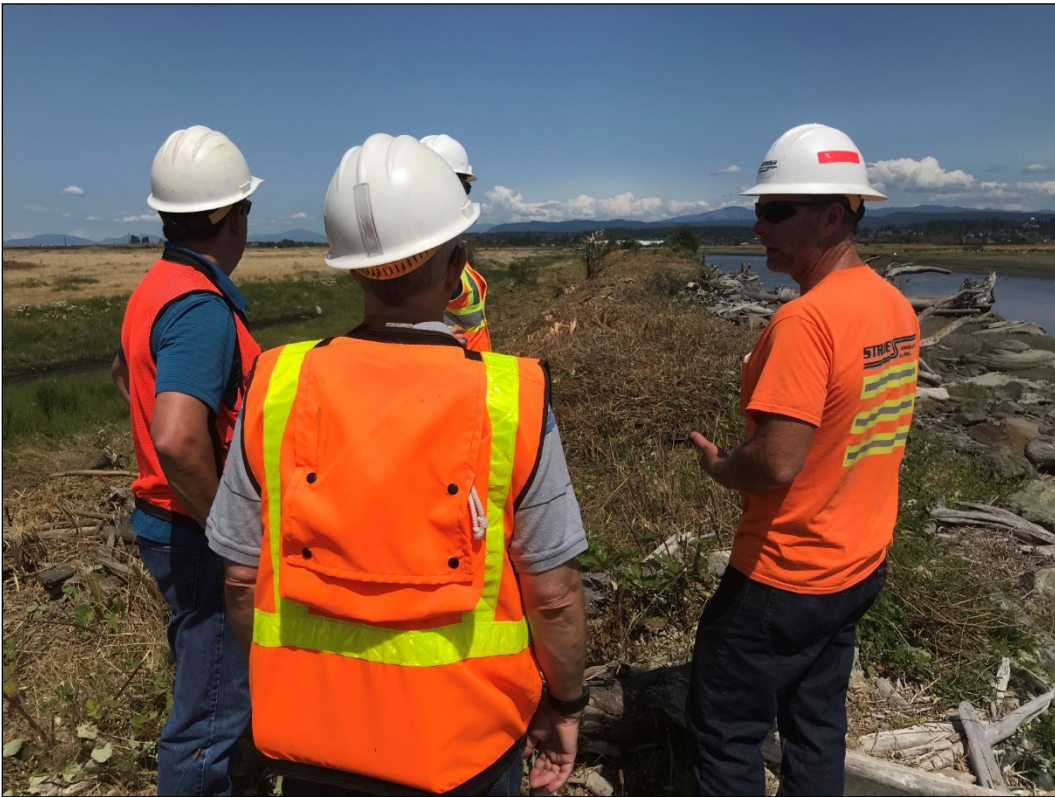
Strider's construction superintendent and the WDFW/Duck's Unlimited project team discuss the plan for dike removal
