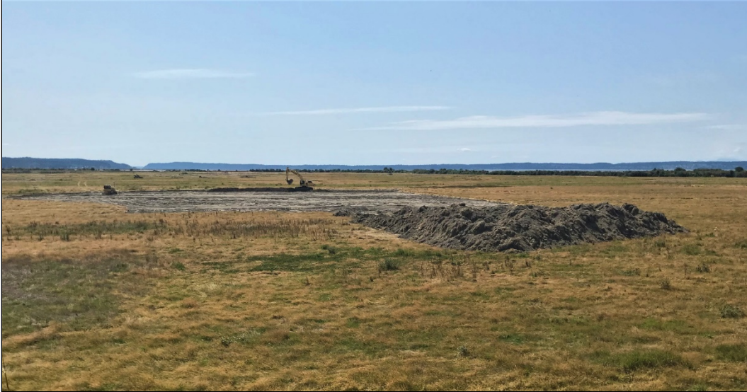
An excavator digs a tidal headwater area on the site that will eventually connected to the tides
