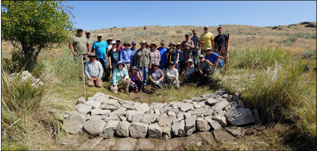
Participants pose after the installation of a one rock dam intended to slow the flow of water, increase bank infiltration, capture sediment, and, over time, raise the channel bed elevation – Photo by J. Maestas
