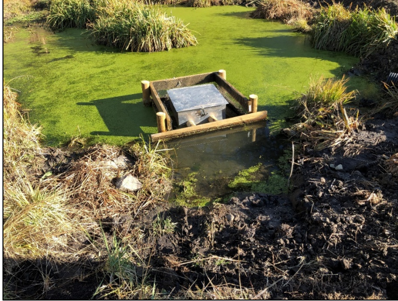
Spring water collection box fabricated and installed by Dave Meisner and Scott McGee
