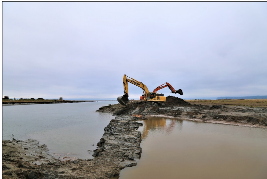
Excavators removed the last ribbon of dirt, connecting 250 acres of Leque Island to Port Susan Bay and the Stillaguamish River
