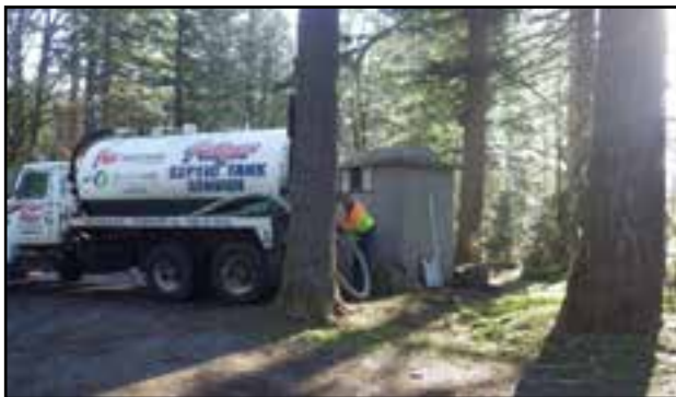
Vault pumping at County Line Access
