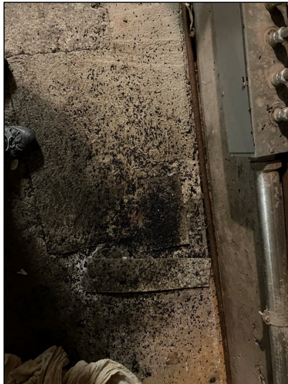
Just one of many locations that bats are dropping guano and roosting inside buildings at Western State Hospital
