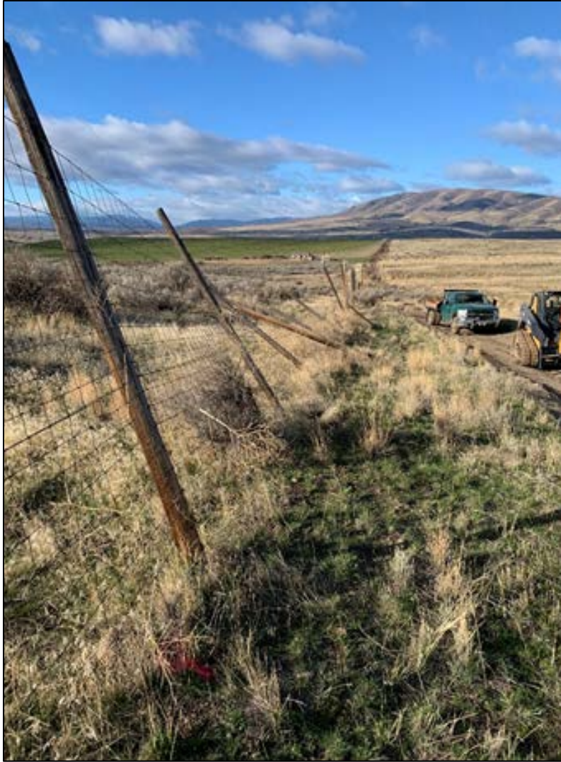
Elk fence being repaired on the Wenas Wildlife Area near Sheep Company Road
