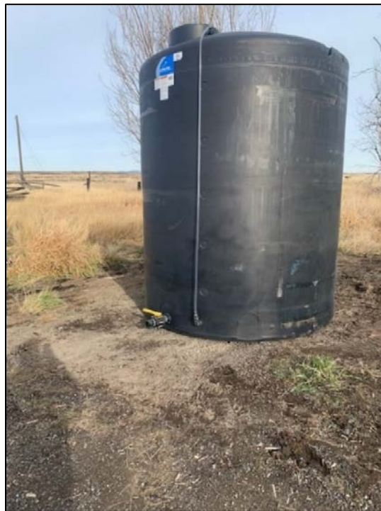
3,000-gallon water tank for Swanson Lakes Wildlife Area
