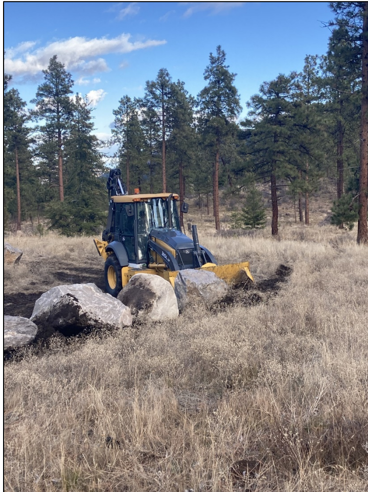
Barrier rock being lined around perimeter of the Lily Lake Snow Park
