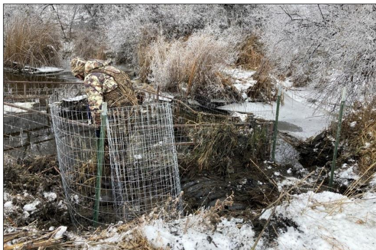
Assistant Manager Ferguson installing new fencing on beaver deceiver at Byron Unit. So far, the beavers have not dammed up the culvert again
