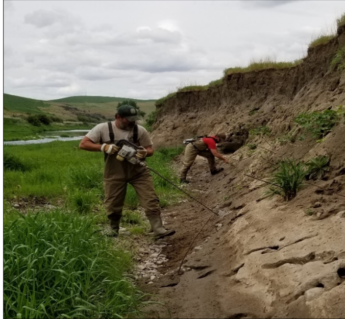
Natural Resource Worker Fish using an auger to make holes for planting
