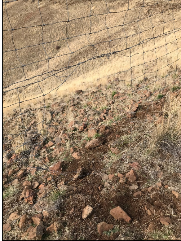
Blown apart wire where elk have been moving through the elk fence above Tum-a-Lum Creek
