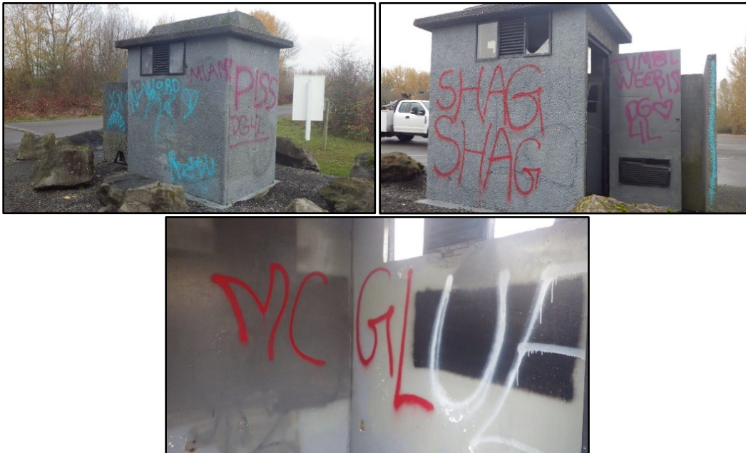
Vancouver Lake Access vandalism
