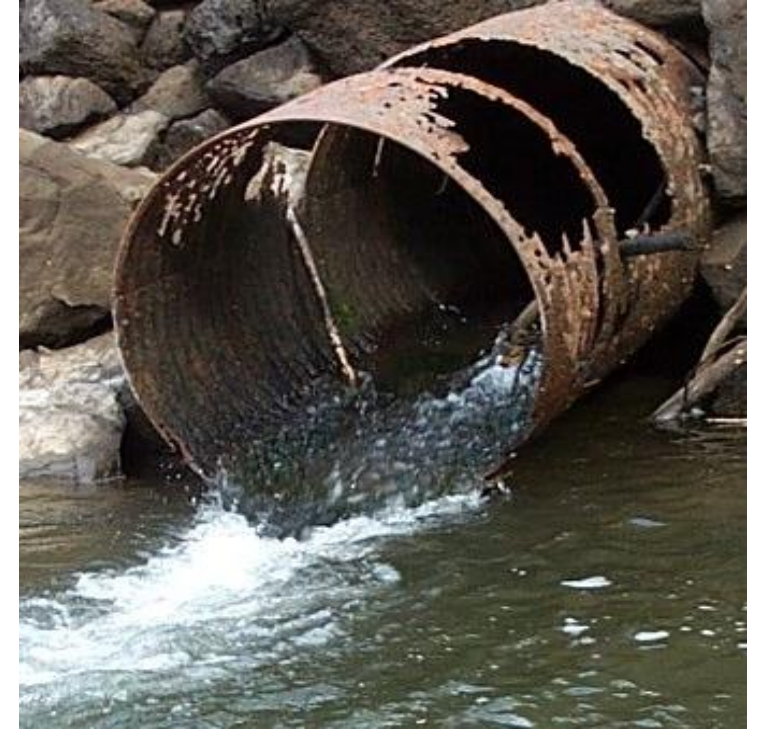
Damage or Deterioration
