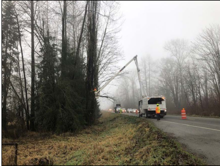
WSDOT and K&D Traffic Services provide traffic control along State Highway 203 while tree work progresses at Cherry Valley
