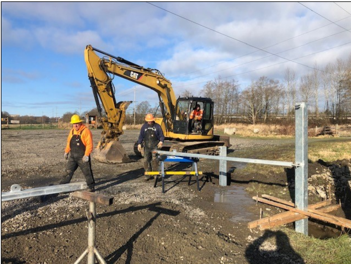
New secured gate being installer at Ebey West parking lot by CAMP
