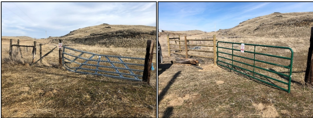
Before and After images of the repaired gate at Horse Spring Coulee Unit – Photo by Wehmeyer
