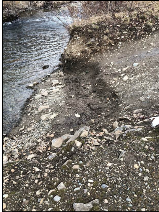
Primitive boat ramp at Teanaway Junction before repair
