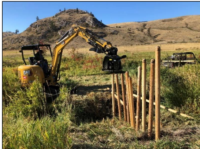
Staff members using a mini excavator and compactor plate to set the posts for the instream structures – Photo by Dupont
