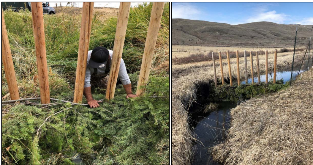
Left to right: Scotch Creek field pro Medina weaving the Douglas Fir branches through the structure and a finished structure in the creek holding water back, lifting the water table, and providing much better conditions for riparian plantings survive and thrive – Photos by Dupont
