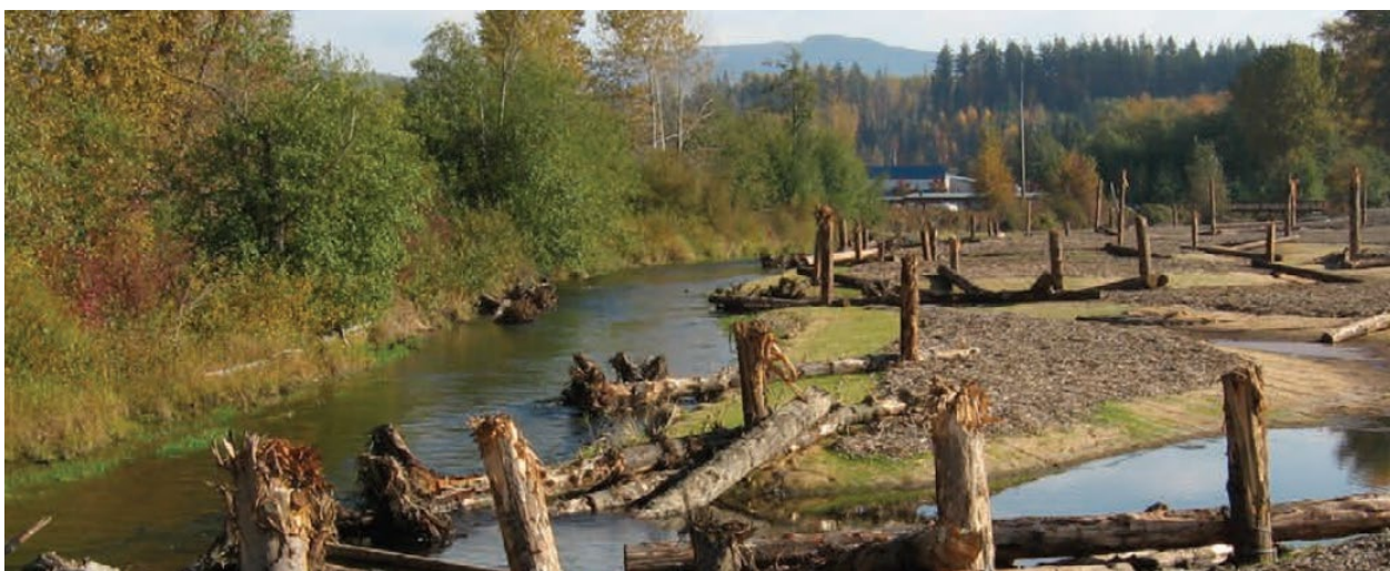
Figure 15: Example of a floodplain reconnection through grading (photo is just after construction). Note the distribution of floodplain and other large wood structures to provide roughness and habitat. | Whatcom Creek, WA
