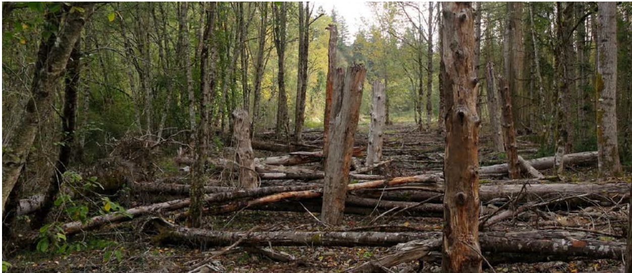
Figure 32: Example of a floodplain roughness large wood used in the decommissioning a temporary construction access route. | Clackamas River, OR
