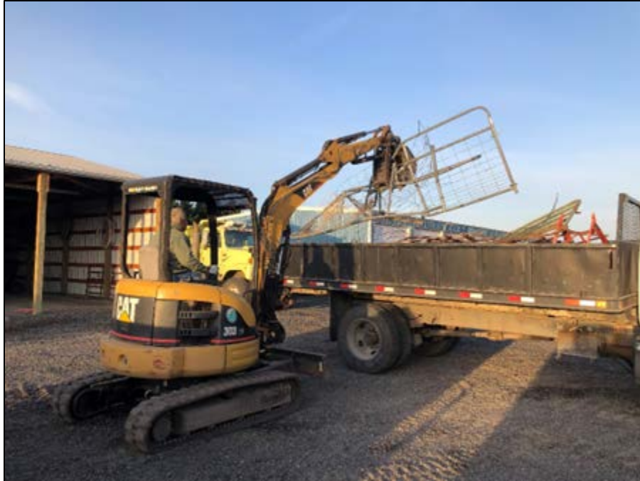
Natural Resource technician Meisner transferring scrap livestock panels from a trailer into our white truck for a final trip to recycling
