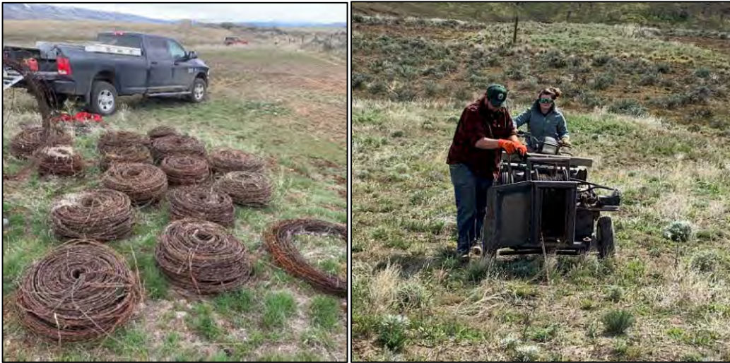
Wire rolled from Mellergaard using mechanical roller. Wire will be staged here and removed in one large load once it has all been rolled. Manager Hughes and Technician Rodriguez rolling wire
