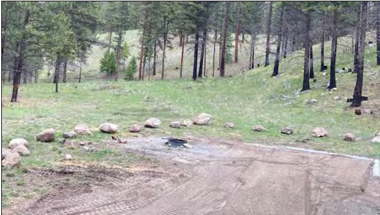
Barrier rock placement within Hunter's Camp on the Sinlahekin – Photo by Wehmeyer
