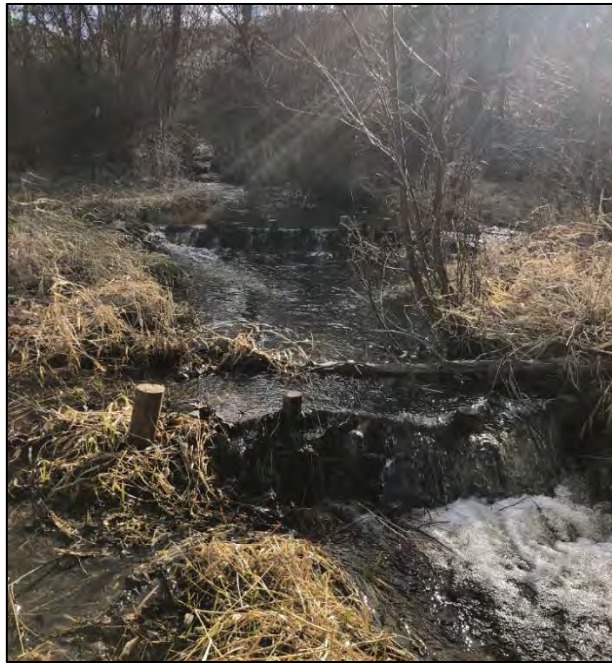
A series of two BDAs installed in 9-mile creek on the Charles and Mary Eder unit by the Colville fish program, spring 2021. The purpose of the BDAs is to slow water flows and recharge the ground water table. Recharging the ground water will increase flows, later in the summer, improving steelhead spawning habitat in the lower portions of the creek – Photo by Dupont
