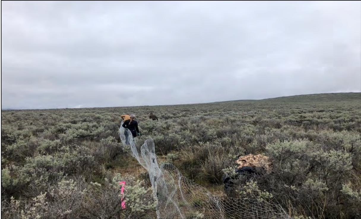
Crew members setting up release pen fencing on the Rimrock Meadows site in Douglas County
