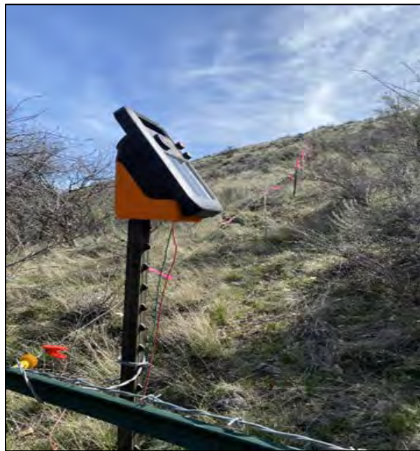
Nass assisted Assistant Manager Winegeart to install temporary fencing to exclude cattle from the re-seeded burn area in the Vantage Pasture, Quilomene, before the grazing period begins next month
