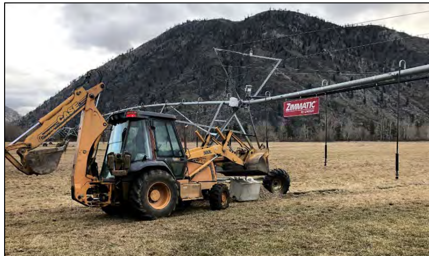
Staff members worked with Chopaka sharecropper Wahl to unload and set the ecology blocks in place at the end of each pivot – Photo by Dupont
