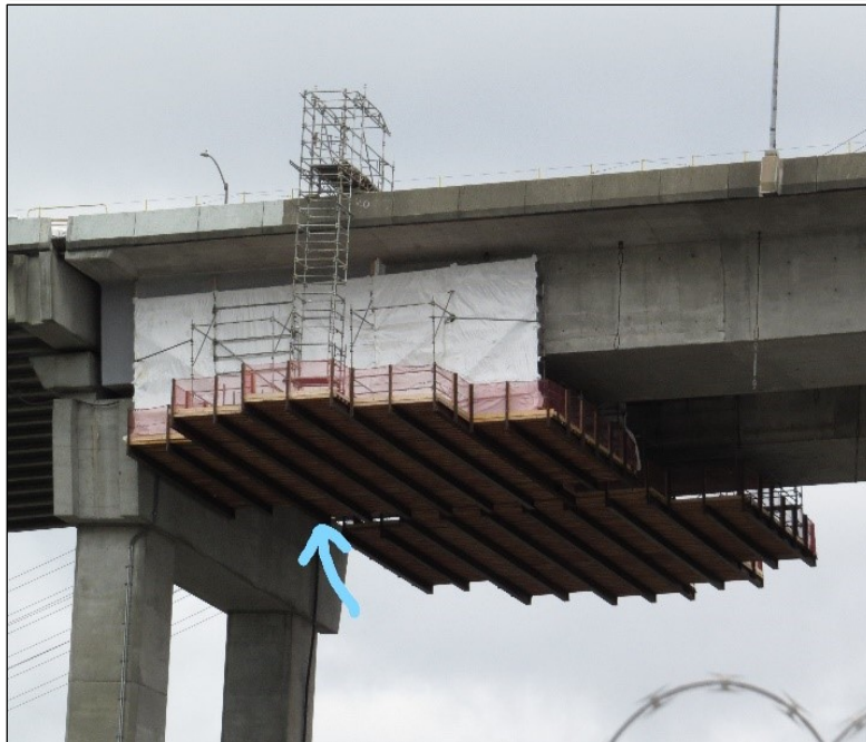
Adult peregrine falcon waiting to relieve partner on nest. Bridge deck work is conducted on hanging platform – the falcon nest is right up in the hanging platform/work site area of the bridge. It definitely took some adjustment on the birds' part but after the Department of Transportation implemented some mitigation measures, things are progressing well and no more divebombing of construction workers now! – Photo by C. Anderson, WDFW
