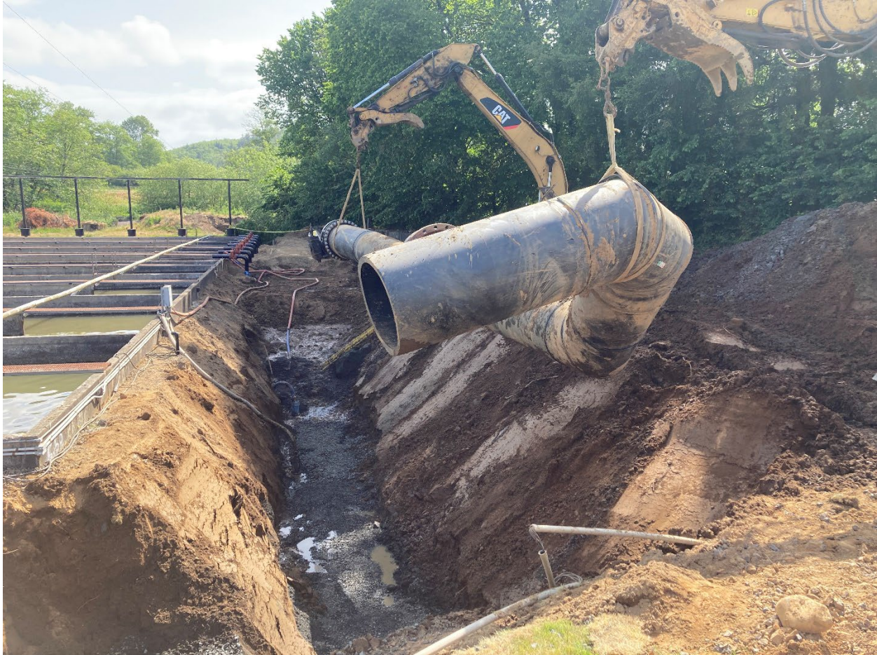
Figure 4: Phase 3 work between areas 1 and 2. Placement of new HDPE line. Earthen pond is behind suspended pipe, in front of vegetation and under dirt at this time.
