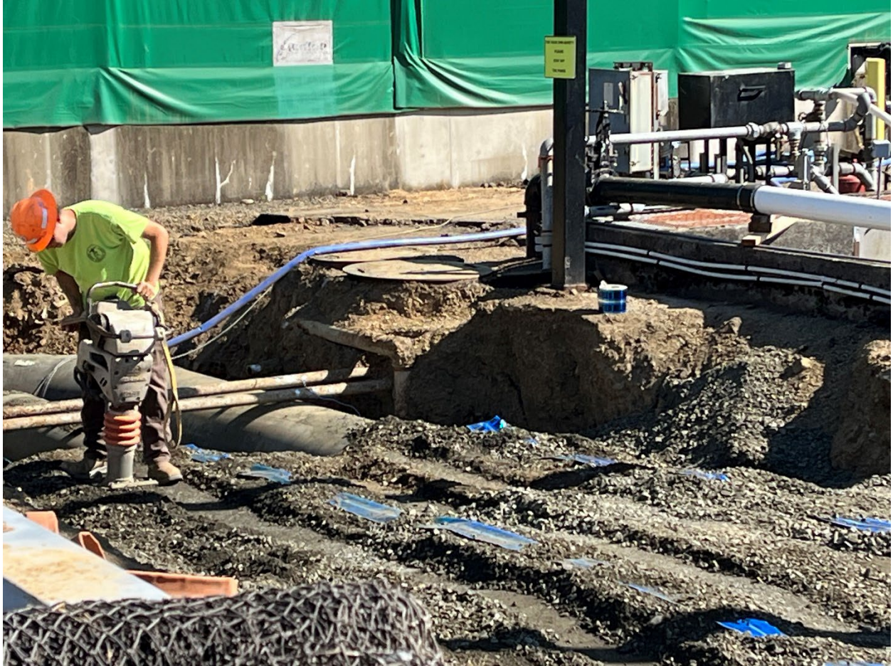
Figure 3: compacting earth around new pipes at hatchery during phase 3 between areas 1 and 2.
