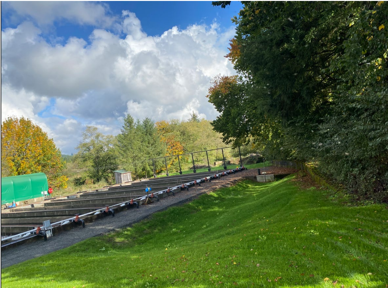
Figure 6: Location of new sediment pond (Phase 4 between areas 1 and 2), currently an earthen pond (the depression). Phase 4, between area 1 and 2. Construction may include some trimming of branches, but no cutting of tree trunks.
