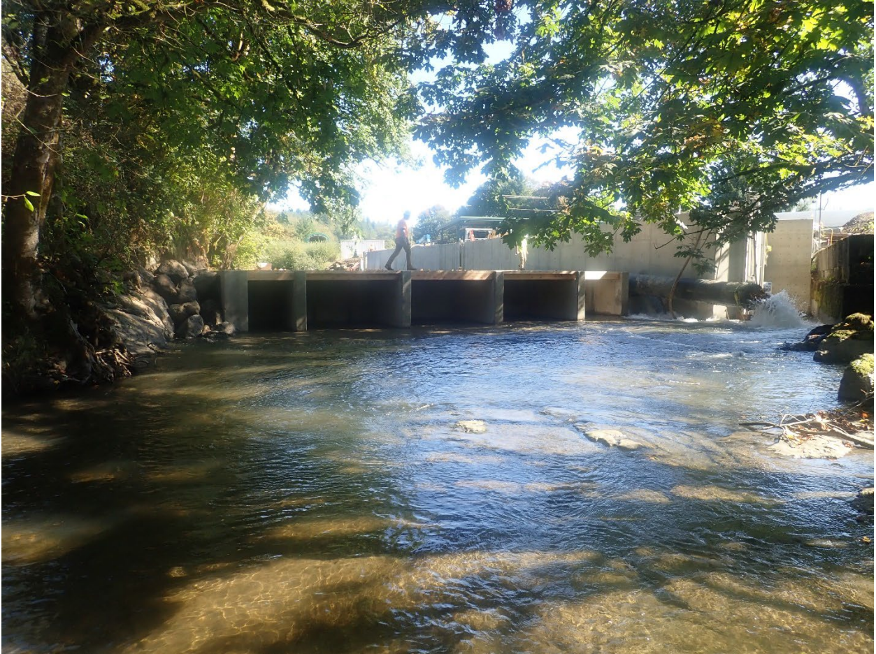
Figure 2: New channel spanning weir at area 1 (person walking across top). New Obermeyer is in slot where pipe is shown in picture.
