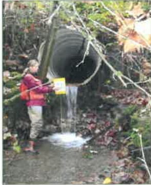
Excessive Water Surface Drop
