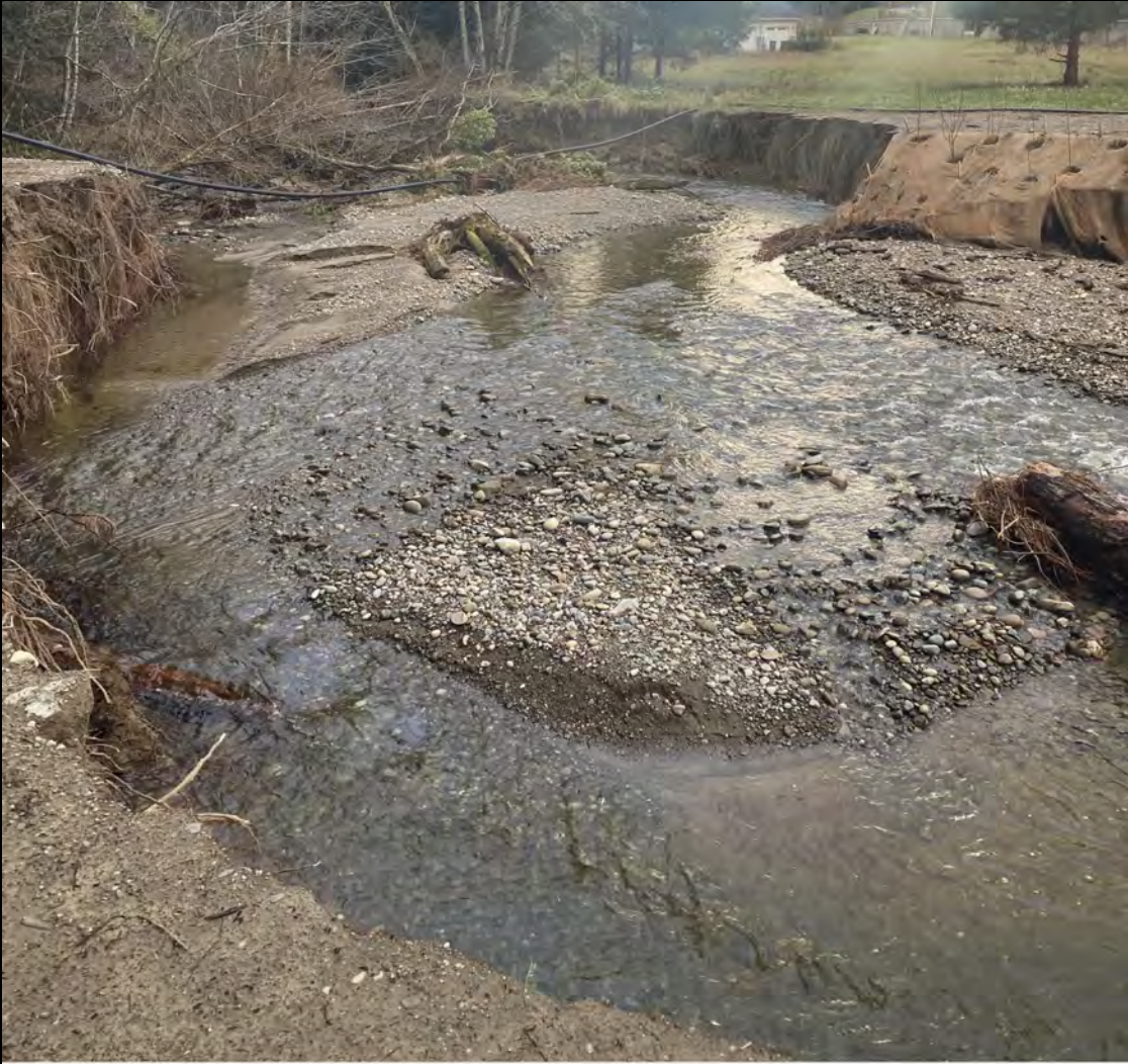
Hood Canal SEG; Seabeck Creek Culvert Replacement (#19-1600) Progress Report: 04/02/2021 Attachment #468368, Seabeck Erosion 1.jpg
