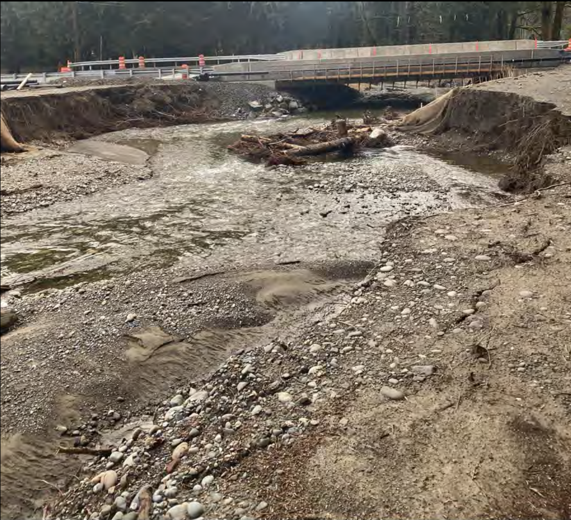
Hood Canal SEG; Seabeck Creek Culvert Replacement (#19-1600) Progress Report: 04/02/2021 Attachment #468369, Seabeck Erosion 2.jpg
