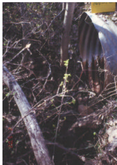
Photo 28. Site 981513 is 2,014 m upstream of the Hutchins Road crossing. This 0.76 m diameter culvert is a total barrier due to slope and outfall drop.
