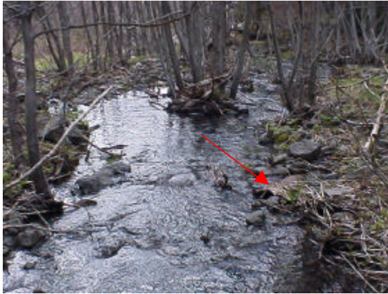
Photo 9. Site 981556, located 867 meters upstream on Whisky Canyon Creek, is passable. The red arrow points to the nearly buried culvert along the right bank.
