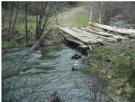
Photo 4. Site 981554 on NF Manastash Creek. The old bridge is currently not a barrier but is deteriorating.
