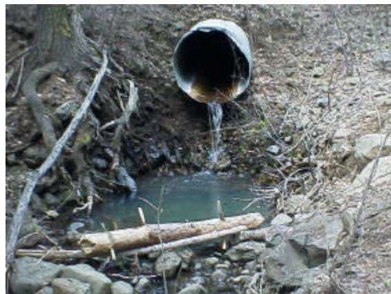
Photo 12. Site 981565, on Whisky Canyon Creek is a 0.91 meter diameter culvert, is a total barrier due to outfall drop and water depth.
