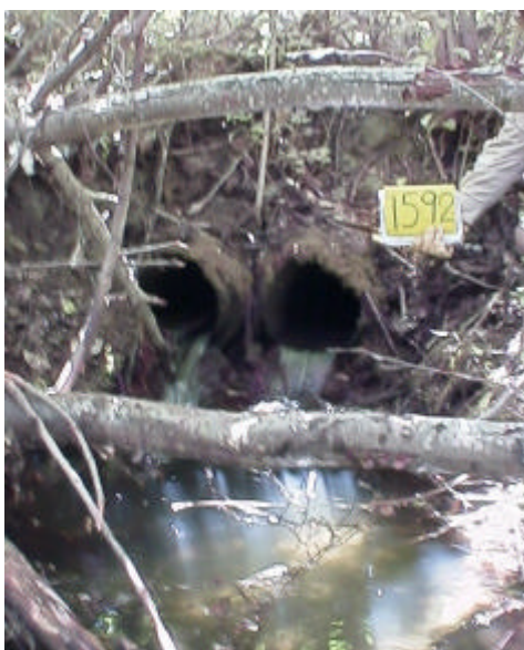
Photo 29. Site 981592, on Yahne Creek, is a pair of 0.31m diameter culverts. This is a partial barrier due to slope and velocity.
