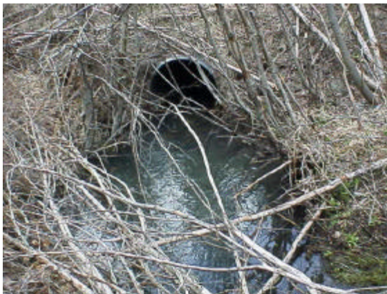
Photo 11. Site 981558, on Whisky Canyon Creek, is a 0.76 meter diameter culvert that is a partial barrier due to velocity and slope.
