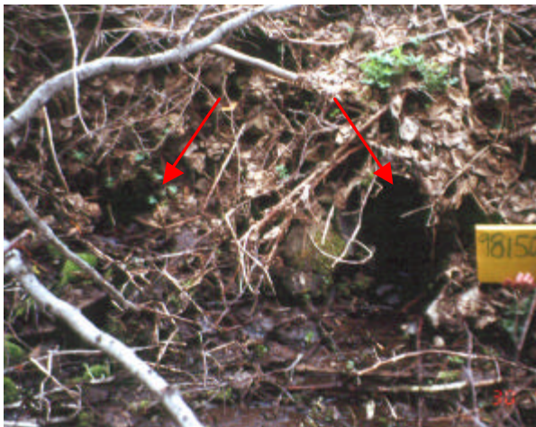
Photo 26. Site 981508 is located on a right bank tributary to Robinson Creek. This pair of 0.46 m diameter culverts are buried at the upstream end, but a small amount of flow seeps through. Most of the stream flows over the road and rejoins the stream channel a short distance downstream.
