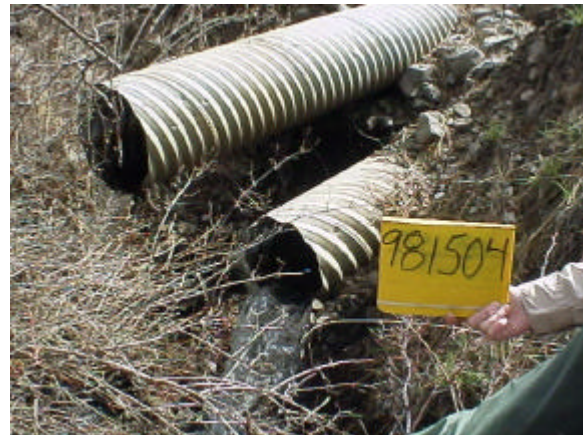
Photo 23. Site 981504, at the mouth of Ainsley Creek, has a pair of perched culverts that are a total barrier to fish passage. This site blocks fish access to 3.2 km of stream.
