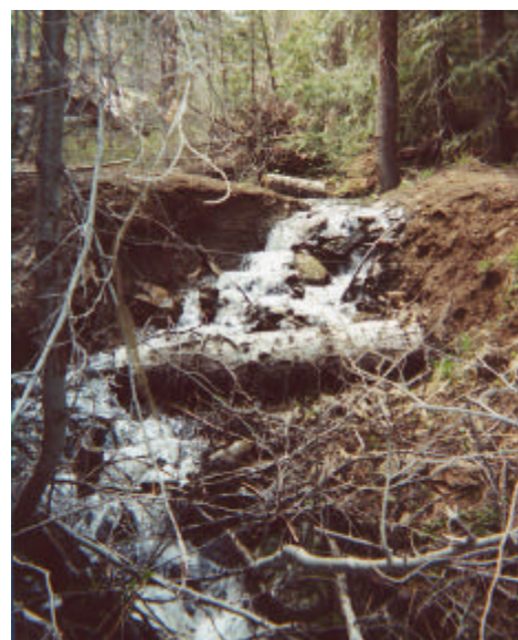
Photo 19. Site 981568, a ford crossing eroding the road. Unnamed tributary to NF Manastash Creek.
