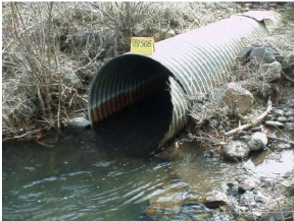
Photo 22. Site 981506, on Robinson Creek, is a 0.91 m diameter culvert that is a partial barrier due velocity and a 2.6% slope. The PI value for this site is 17.17.
