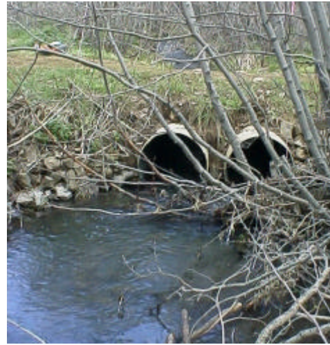
Photo 17. Site 981571, is 944 meters upstream on an unnamed tributary to NF Manastash Creek. A pair of 0.61 m diameter culverts create a partial barrier due to a 4.6% slope. This site is on Murray Road.
