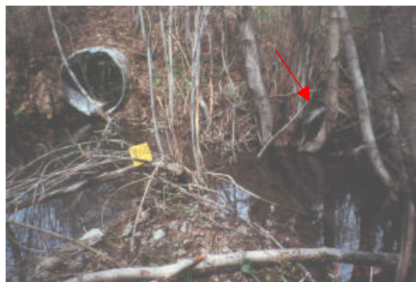
Photo 25. Site 981522 on Ainsley Creek. The red arrow points to a 0.61m diameter culvert. The culvert on the left is a 0.91m diameter overflow culvert.
