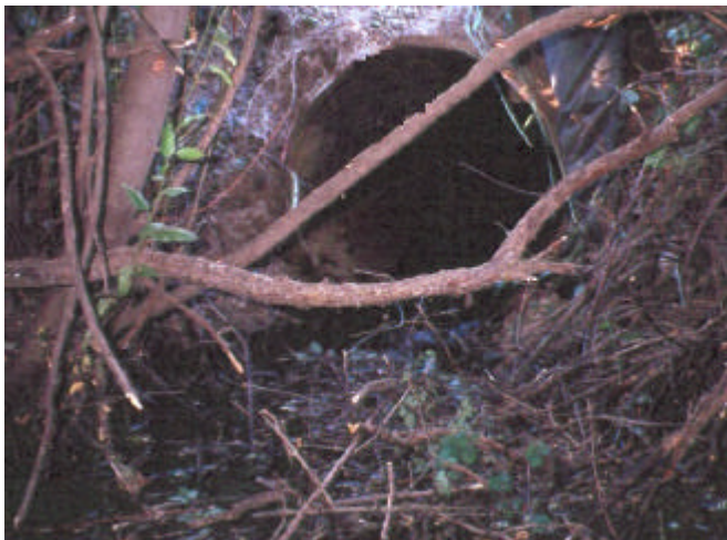
Photo 27. Site 981514 is located on Joe Watt Creek where it crosses Hutchins Road. This 0.76 m diameter culvert is a partial barrier due to slope.
