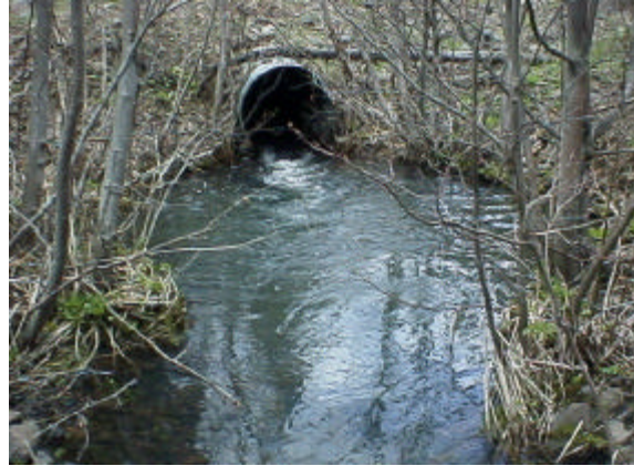
Photo 10. Site 981557, on Whisky Canyon Creek, is a 0.76 meter diameter culvert. This undersized culvert is a total barrier due to velocity and a 6% slope.
