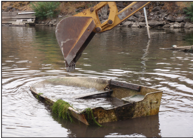
An excavator removes a sunken boat as part of a clean-up project on the lower White Salmon river
