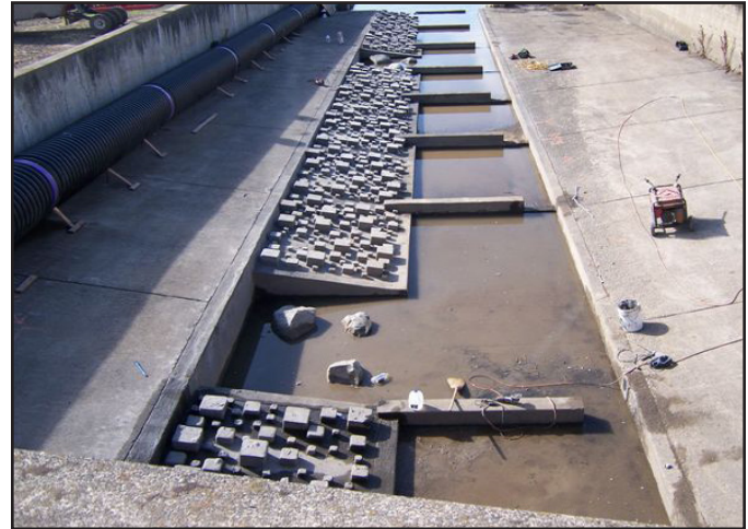
Precast roughness panels and a resting pool will improve fish passage in the Mill Creek flood control channel.
