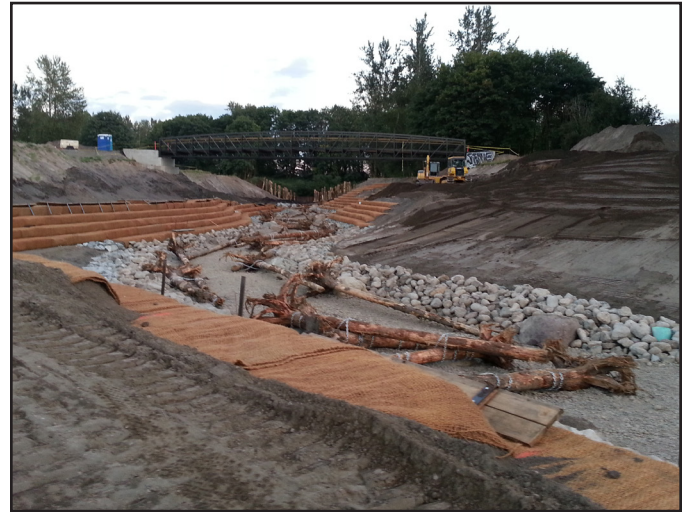
Looking upstream at new side channel construction at Riverview Park on the Green River
