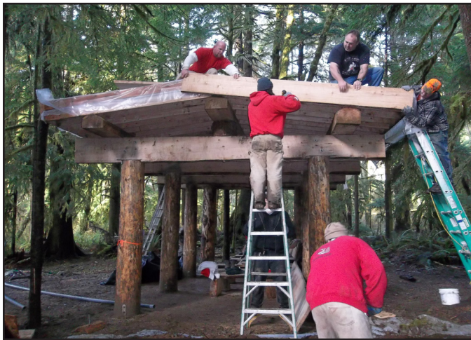
Staff, volunteers and DOC crew putting fascia on the Elk Creek "Ed Shed"
