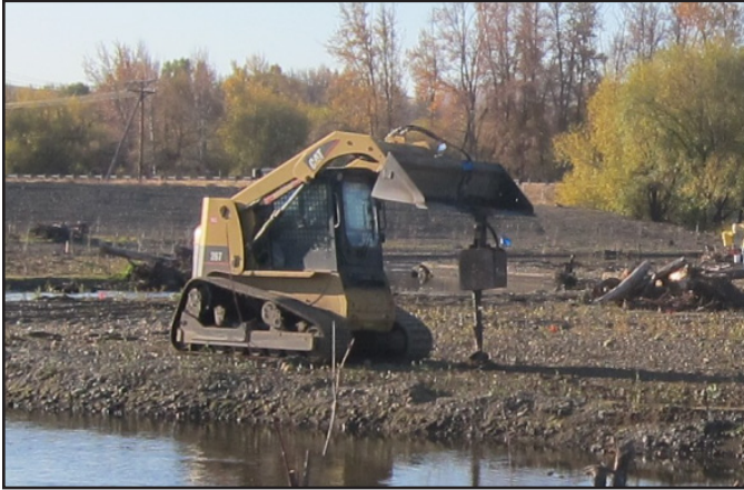
A bobcat with an auger attachment digs holes for riparian planting at the Reecer Creek Floodplain Restoration project in Ellensburg.
