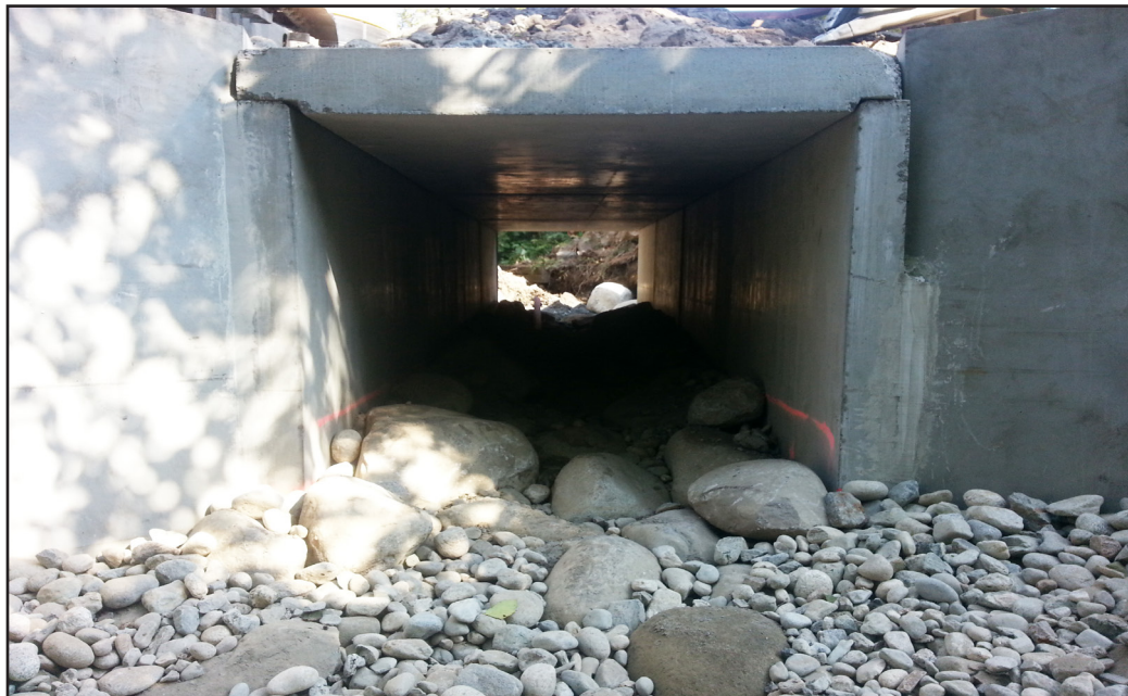
New Culvert installed at Little Brook Creek with boulder cascade stream bed constructed inside.
