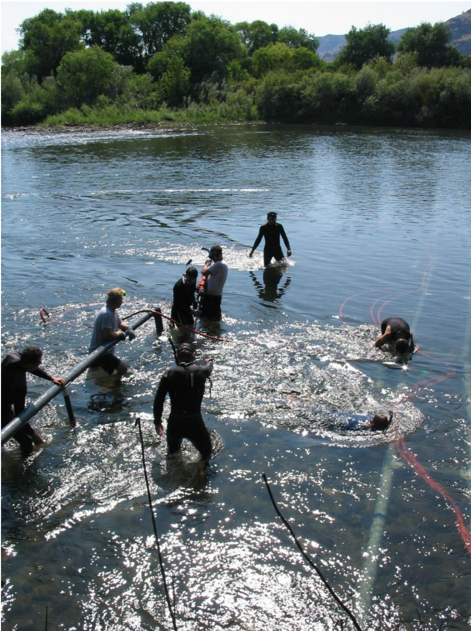
Figure 1. PIT tag antennas being installed in the Okanogan River by Washington Department of Fish and Wildlife and Colville Confederated Tribes Fish and Wildlife staff in September 2013.
