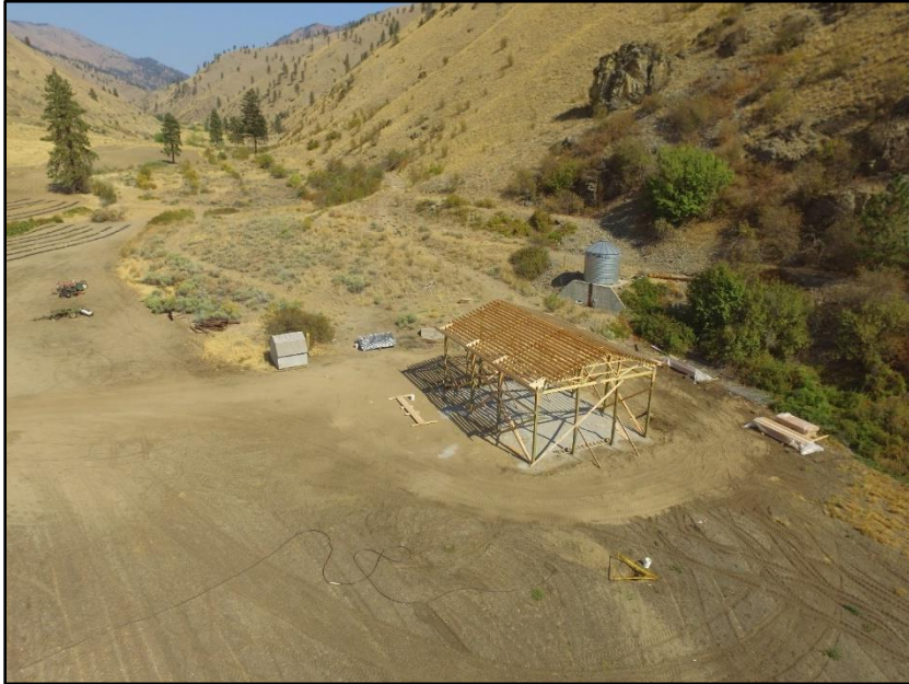
Swakane storage / shop building – Photo by Daniel Hammerstrom, Glacier Industries
