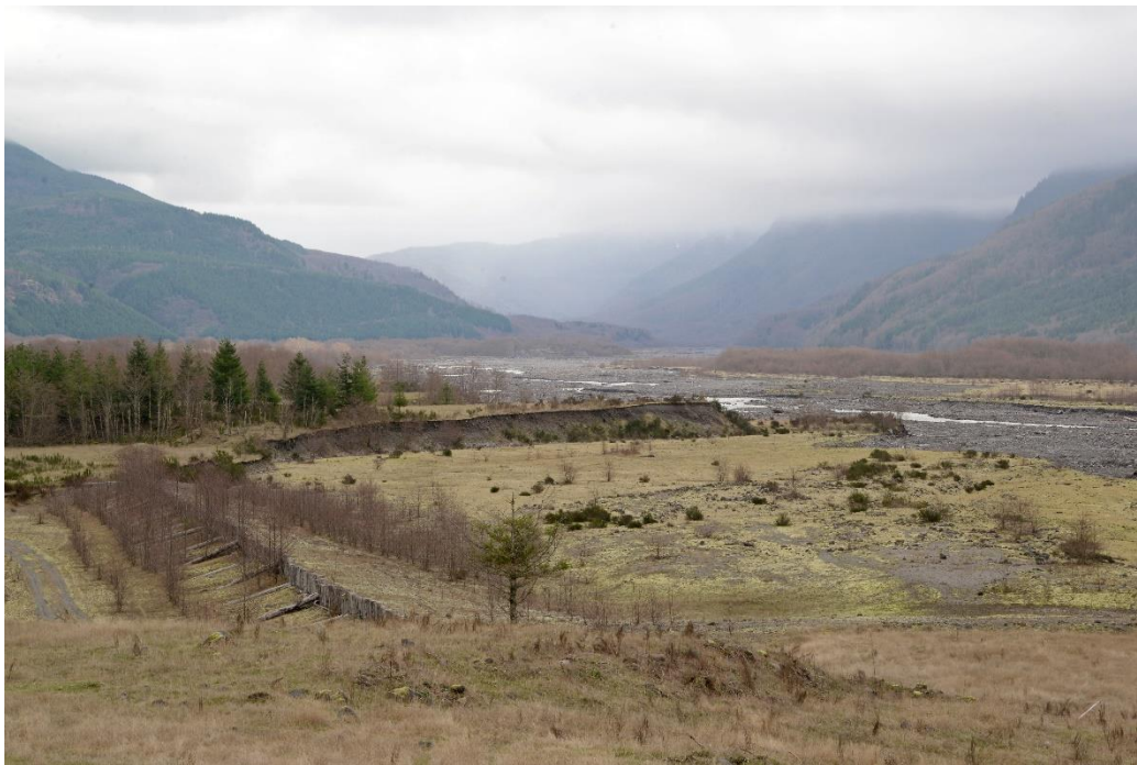
Mudflow Unit – Toutle River – erosion control work. Photo by Alan L. Bauer.
