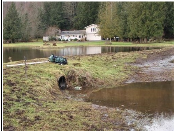
A full span earthen fill dam with culvert outlet. The culvert is intentionally perched on the upstream end to impound water.
