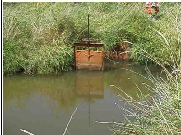
A screw gate at the upstream end of a culvert, resulting in a dam feature.
