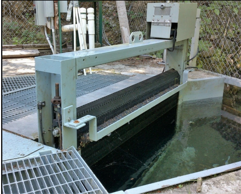
Figure 9.5. A photograph of a traveling belt screen.
