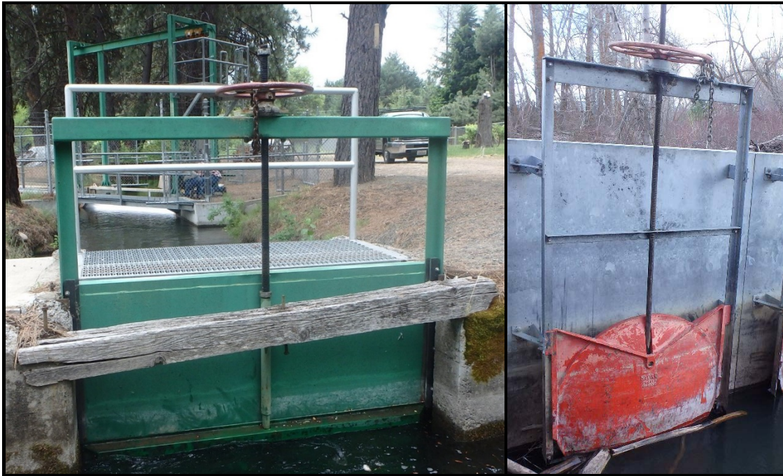
Figure 9.3. Examples of diversion headgate designs. The pictures above show two examples of headgates that may be associated with surface water diversions.
