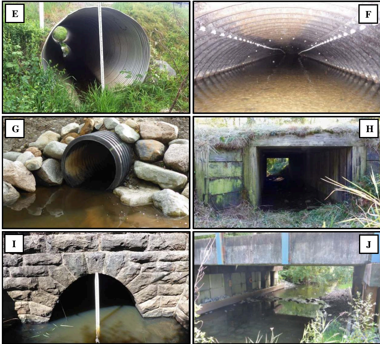
Figure 3.5 (Continued). Examples of culvert construction materials. E) Corrugated Aluminum (CAL), F) Structural Plate Steel (SPS), G) Plastic (PVC), H) Timber (TMB), I) Masonry (MRY), J) Other (OTH)
