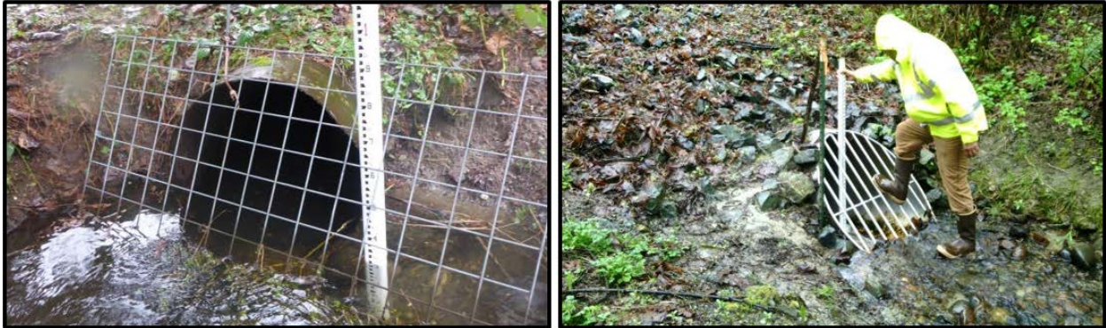
Figure 3.15. Examples of culverts with racks. Note: stadia rods are in the pictures for scale only. They do not illustrate where to measure rack dimensions.
