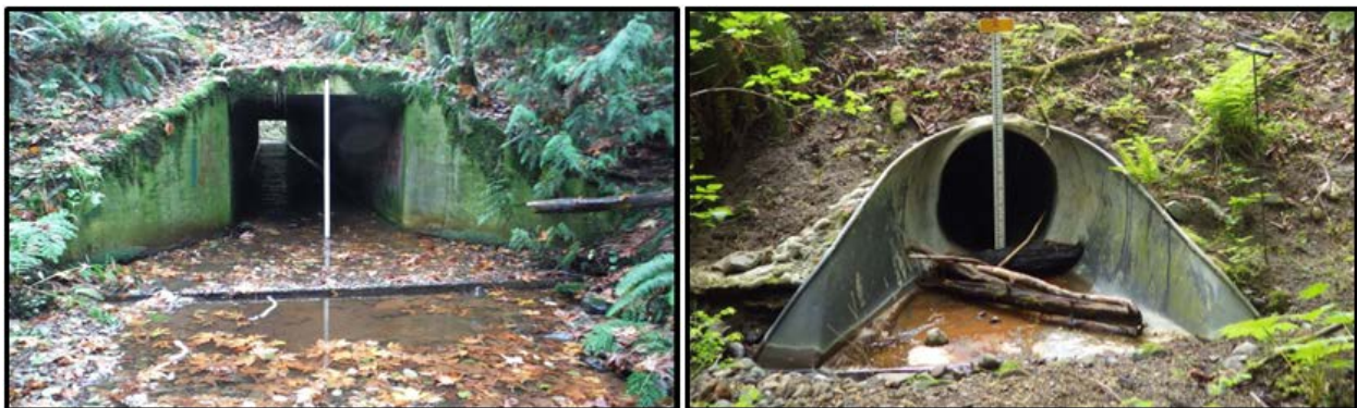
Figure 3.9. Examples of aprons. Locate the ends of any aprons to include in the measurements of total length and culvert slope. The left image illustrates an apron at downstream end of a box culvert. The right image illustrates an apron at upstream end of a round culvert.
