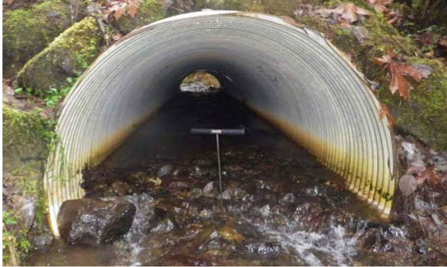
Figure 3.12. Countersunk culvert. A tile probe is used to determine if the culvert outlet invert is embedded at a depth \geq 20\% of the culvert rise.
