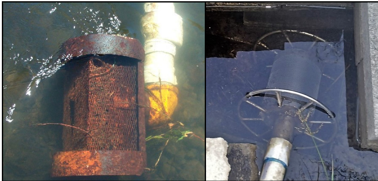
Figure 9.11. Photographs of pump screens.
