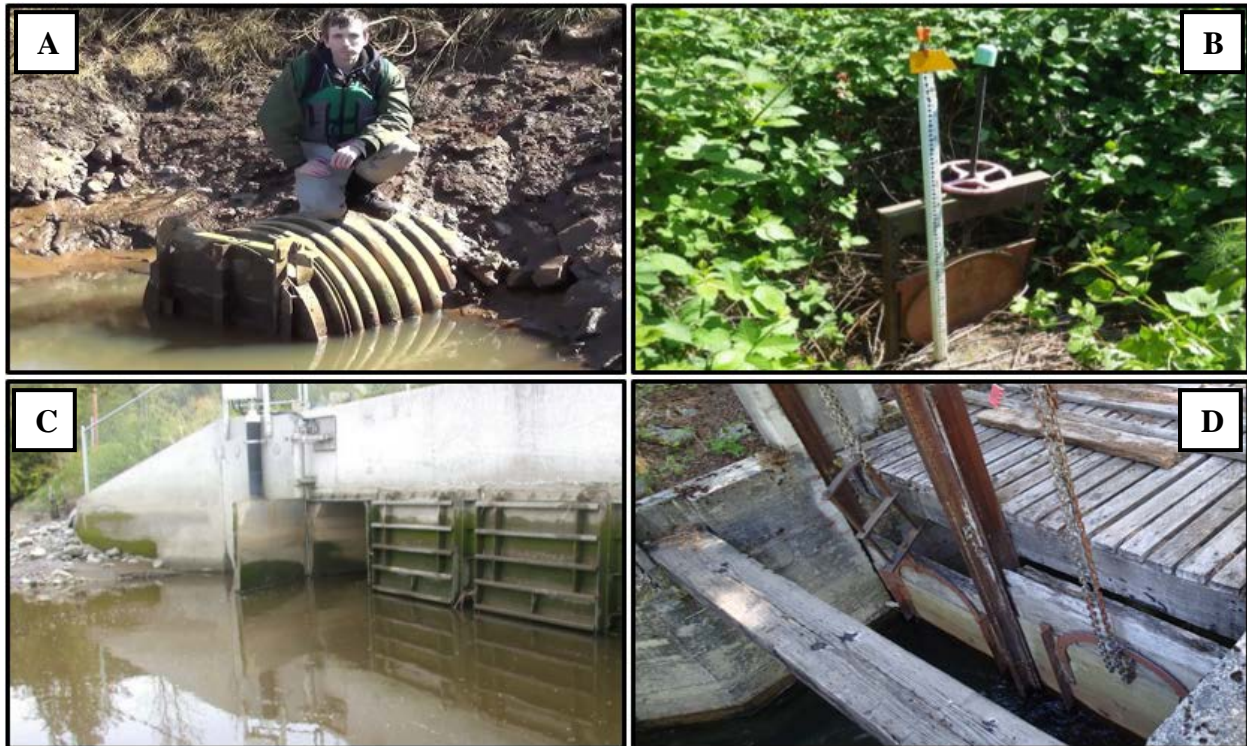
Figure 3.14. Examples of culverts with gates. A) Flap gate, B) Screw gate, C) Swing gate, D) Slide gate.
