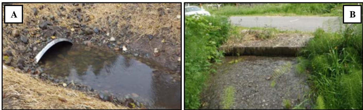
Figure 3.13. Culverts with excess bed material. When there is a substantial loss of hydraulic capacity and headroom, the Level A flowchart (Figure 3.19) and multiple culvert key (Box 3.2) may not be applicable to the barrier determination. A) if there is a significant loss in hydraulic capacity but the headroom is still \geq 0.30 meters, use the Level B hydraulic analysis to estimate velocity. B) if headroom < 0.30 meters, then the culvert is considered a barrier due to lack of headroom.
